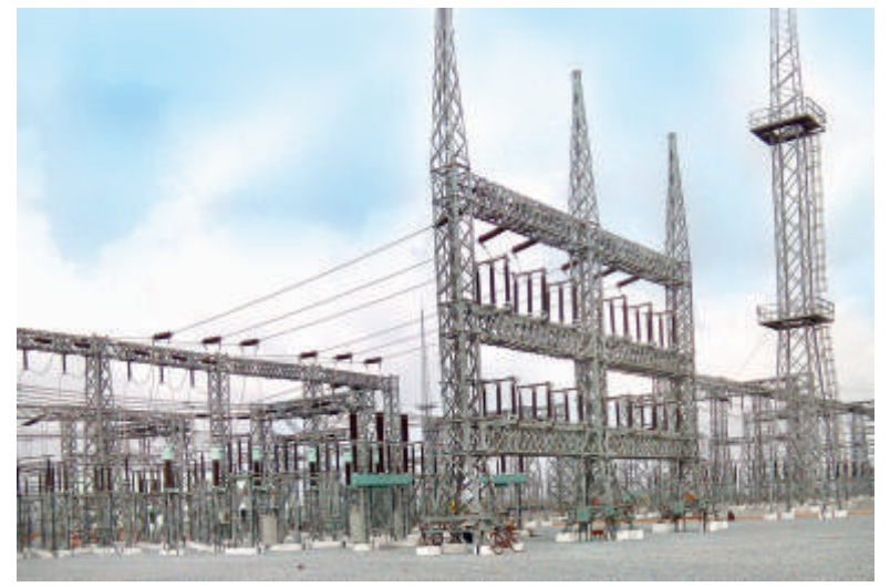
400 KV Substation Thervaikandigai, TANTRANSO - Tamilnadu.
