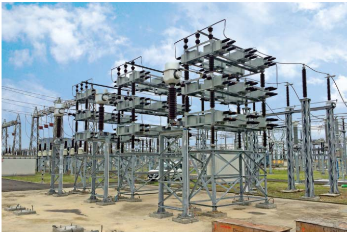
54 MVAR, 132 KV TERNA Rete, Italy.
