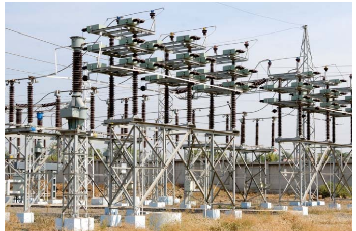
132 KV Fuseless Capacitor Bank, Phaltan, Maharashtra, MSETCL
