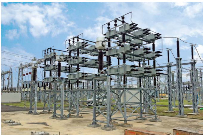
54 MVAR, 132 KV TERNA Rete, Italy.
