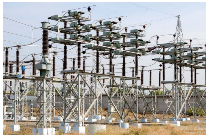
132 KV Fuseless Capacitor Bank, Phaltan, Maharashtra, MSETCL
